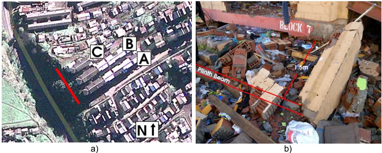
Figure 20. Collapse of a three-story confined masonry building in Constitución, Chile due to the February 2010 Maule earthquake: a) an aerial view of buildings A, B and C (note a steep slope on the north-west side shown with a solid line), and b) building C (located closest to the slope) lost the ground floor and moved by approximately 1.5 m away from the plinth towards north (S. Brzev).
