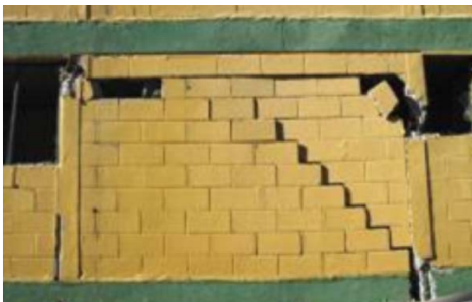
Figure 8. Critical regions in a confined masonry building: a) a general diagram showing critical regions in the RC tie-columns, and b) tie-column damage observed in the 2010 Chile earthquake (M. Astroza).
