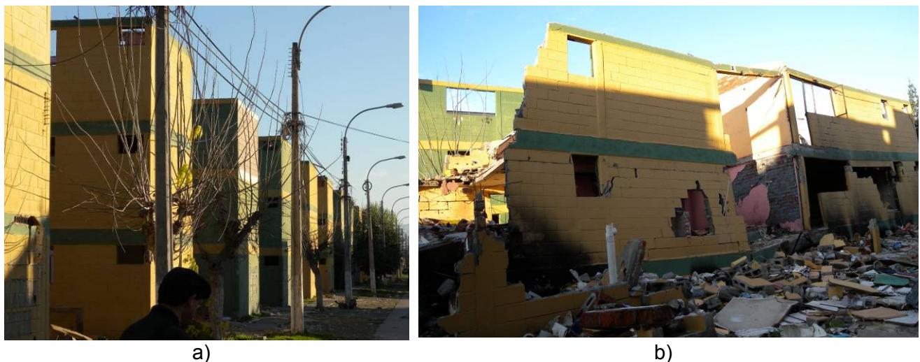
Figure 19. Collapse of a three-story confined masonry building in Santa Cruz, Chile due to the February 2010 Maule earthquake: a) building complex, and b) a building that experienced collapse at the ground floor level (S. Brzev).
