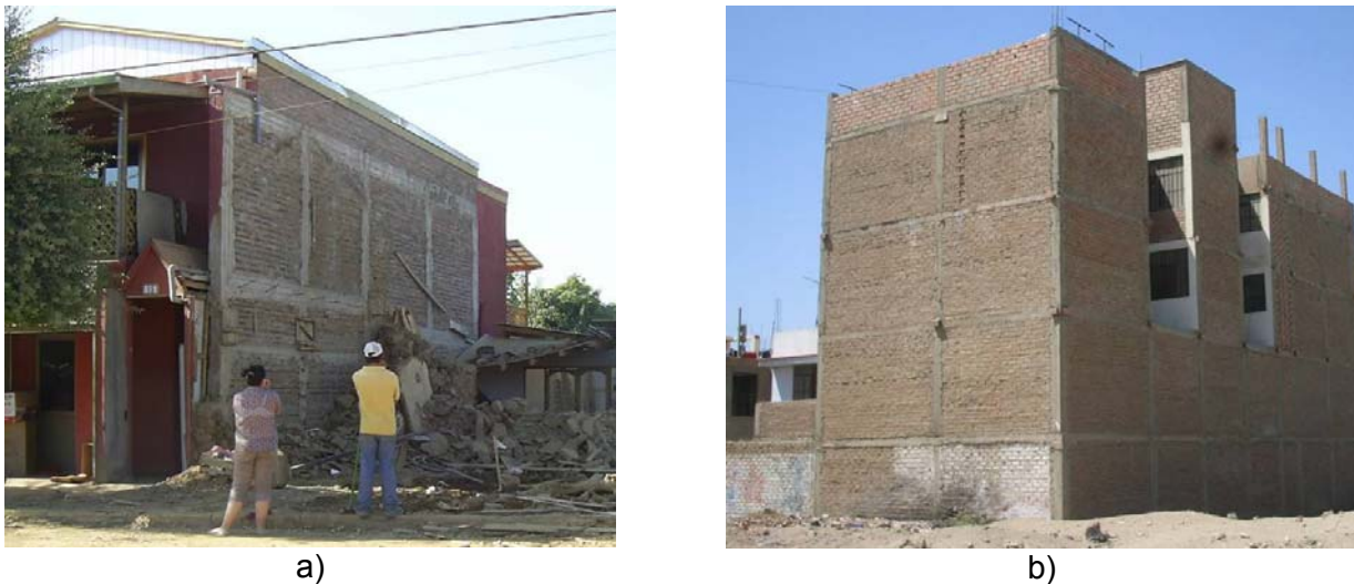
Figure 4. Performance of confined masonry buildings in recent significant earthquakes: a) the 2010 Maule, Chile earthquake (M.O. Moroni Yadlin), and b) the 2007 Pisco, Peru earthquake (D. Quiun).
